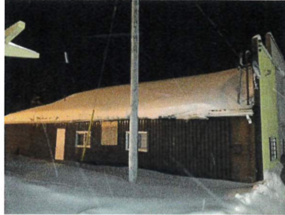
Photo 14: Potential ACM caulking and/or sealants around windows, doors and roof-mounted equipment – Exterior.
