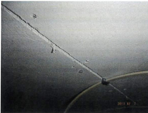
Photo 7: AC grey fibrous ceiling boards above the CTs (HCH - S7) - Room #6 - Mens' washroom.
