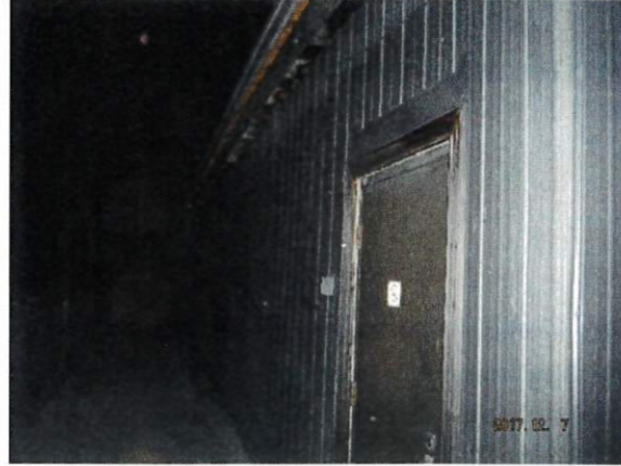
Photo 17: Potential ACM insulating materials inside hollow metal doors – Throughout subject building.
