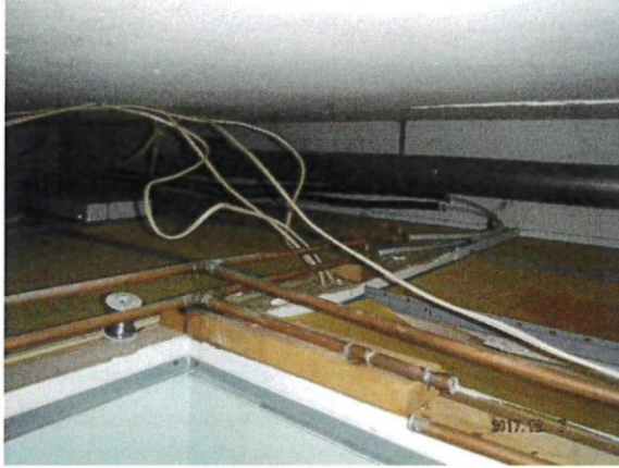
Photo 16: Uninsulated piping and ductwork observed throughout the building.
