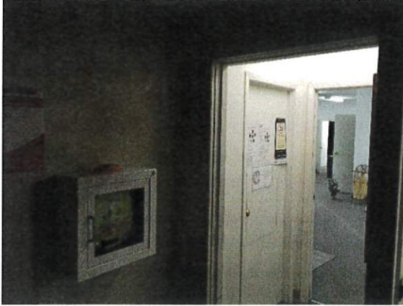
Photo 13: Potential ACM insulation materials inside hollow metal doors – Throughout subject building.
